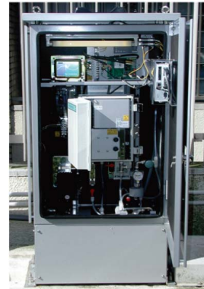
Water Quality Telemeter
