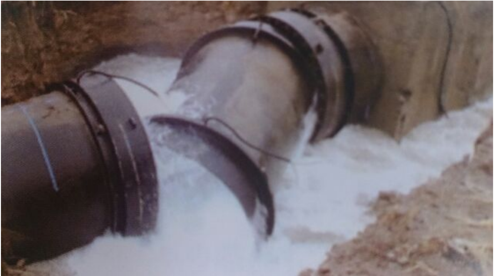
Slip-Out of Transmission Mains ( \phi 2400\text{mm} )
