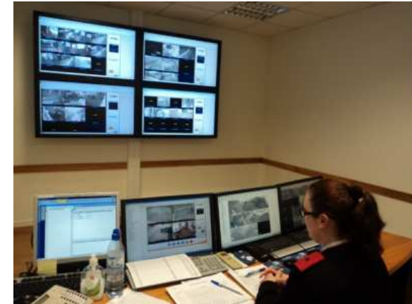
Security Command and Control Center
